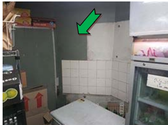
Photo 4. Interior, storage room, walls – non asbestos-containing fibre cement sheeting and suspected lead-containing green upper paint systems.
