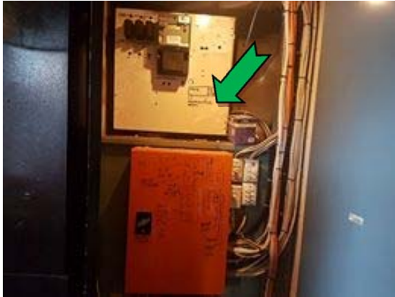
Photo 1. Interior, south-west elevation, electrical distribution cupboard, electrical backing board – suspected non asbestos-containing bituminous backing board.
